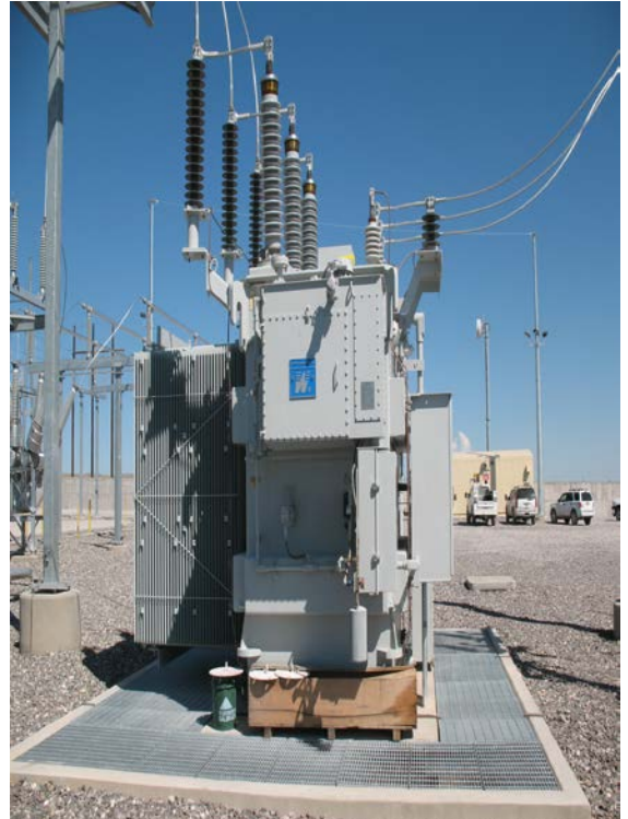
10 MVA Power Transformer at the Frontier Substation.
